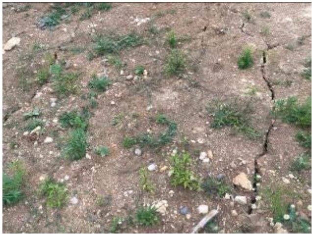
Cracks on the ground surface at the spoil disposal area (landslide hazard)
